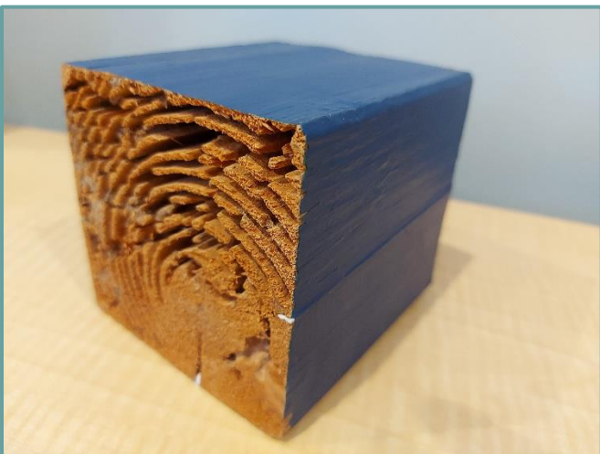
Section from a destroyed verandah post. Note the zero evidence on the exterior.
